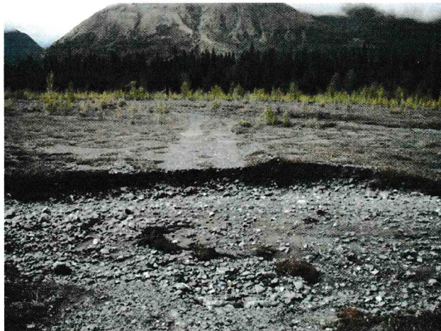
Plate 1: Washout on access trail
